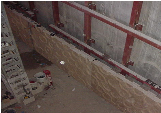
Hoist was used in the install of an art wall at MIA.
